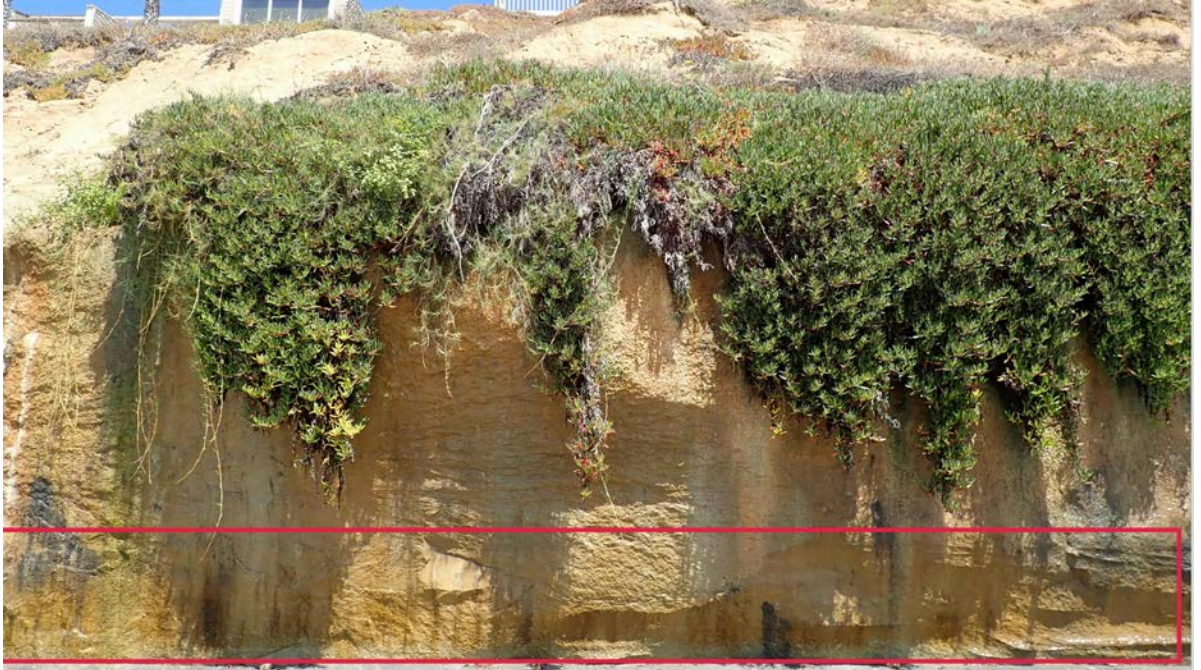
Subject cliff collapse site: undercutting of cliff
